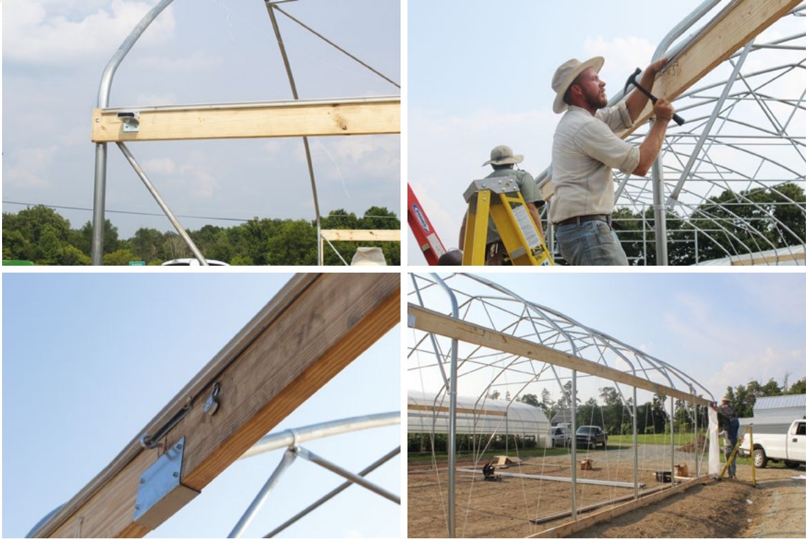
Picture 2-9: Installing anchors, hooks and pulleys on the hip board, inserting steel cords through the hooks, and then nailing the nylon string on the hip board and base board.
