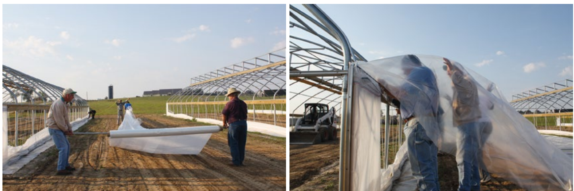
Picture 2-14: Laying plastic film on the ground and securing the plastic film to the c-channels on the hip board with wiggle wires.
