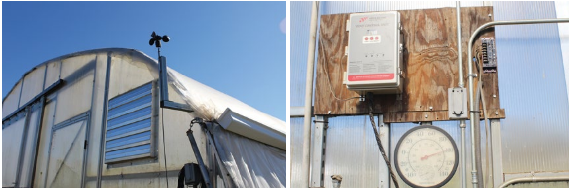
Picture 8-4: A wind and temperature controlled automatic ventilation system at an N.C. A&T University Farm high tunnel. Wind speeds that exceed the set-up threshold, for example 25 miles/hour, will override the temperature control thus protecting the plastic cover.
