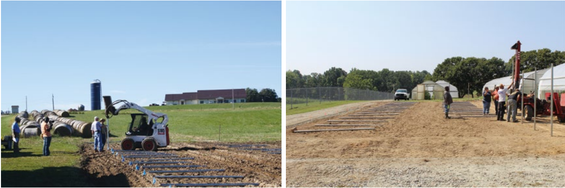
Picture 2-3: Installing side wall posts using a post driver. Left: a post driver for 6-foot or less tall side wall posts; Right: a post driver for side wall posts that are taller than six feet.
