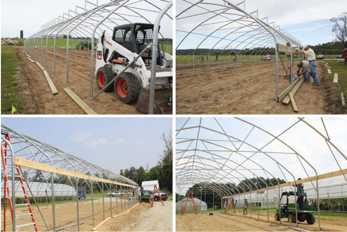
Picture 2-7: Laying out base and hip boards and attaching them to the side posts (upper); Installation of hip and base boards completed (lower).
