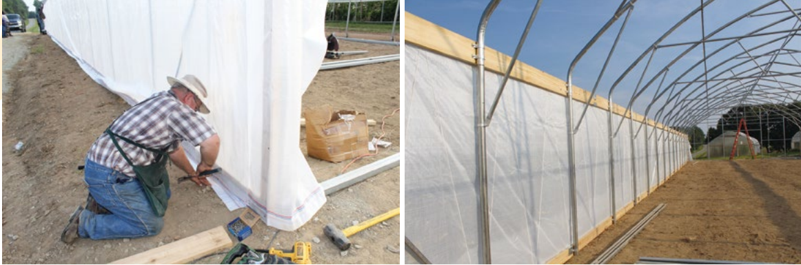
Picture 2-11: Nailing the lower side of the curtain to the base board (left). A completed side curtain (right) after installing the outside protecting nylon strings.
