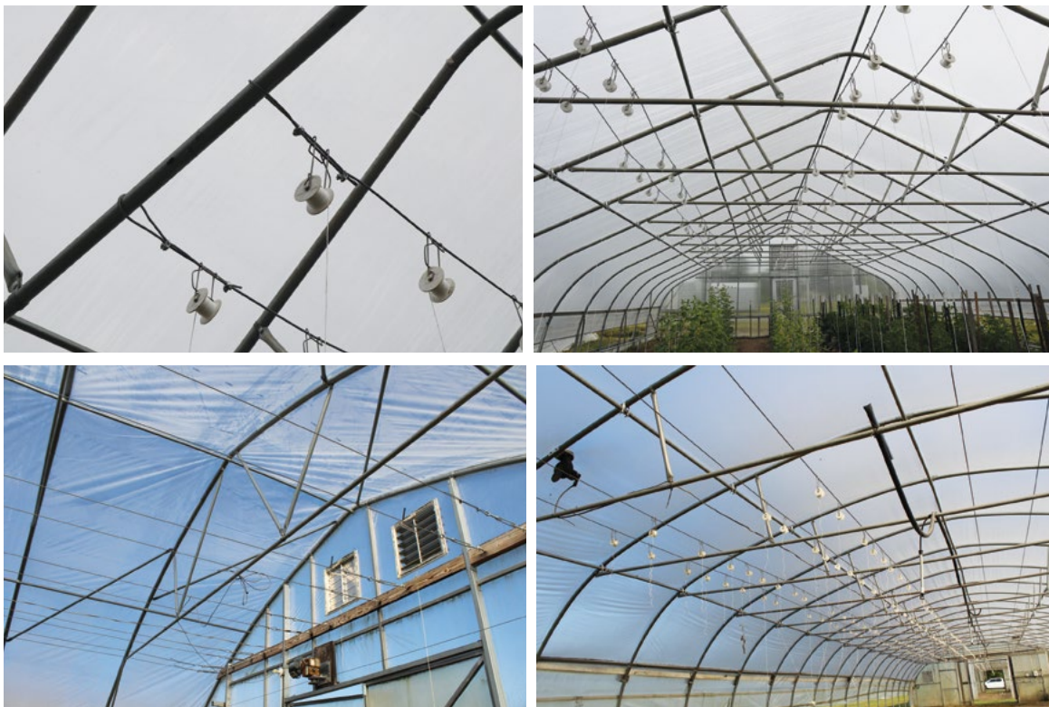
Picture 6-4. Braces in high tunnels are used to support wires for the Roller-Hook® trellis system (top). Anchor boards can also be added to end walls for support of trellises (bottom).
