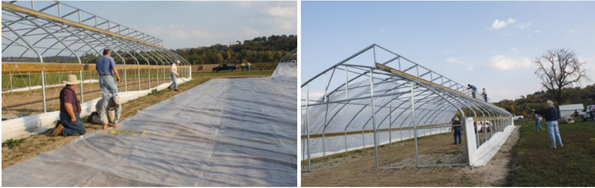
Picture 2-15: Tying the plastic film and pulling the rope to pull the plastic film over the roof.
