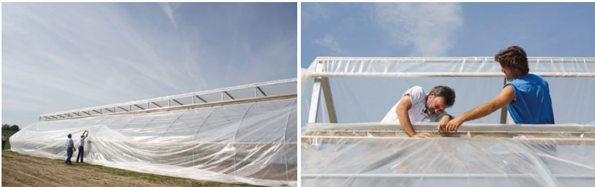
Picture 2-17: Putting on the second layer of plastic film if your high tunnel has double-layer plastic cover.
