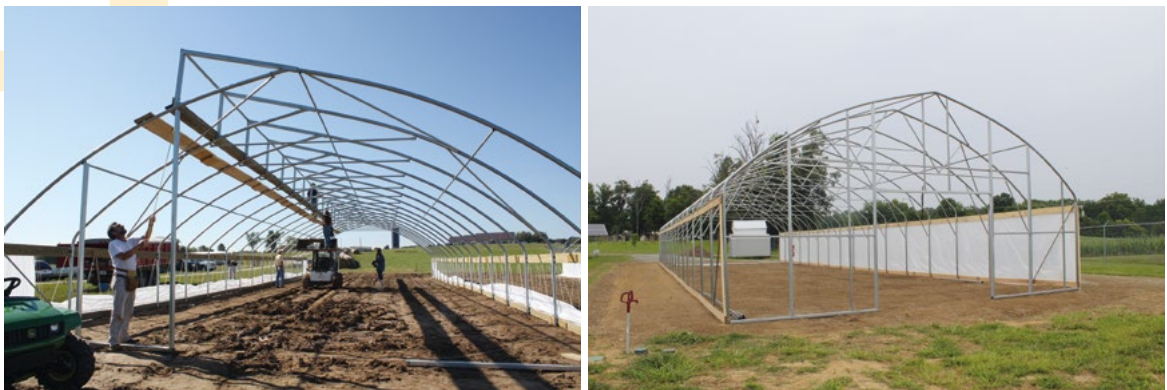
Picture 2-13: Constructing end walls. Left, on-site measuring for the length of vertical bars; Right, a completed end wall frame.
