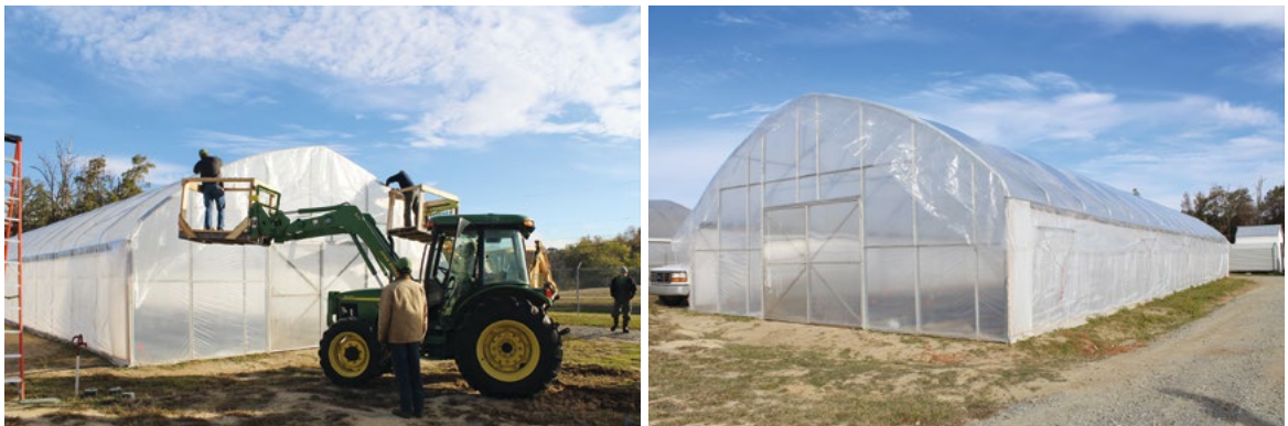
Picture 2-19: Putting plastic on end walls for a high tunnel without a ridge vent.
